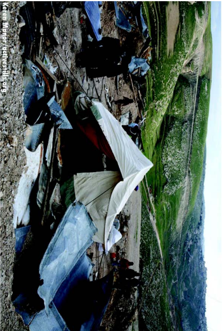
Demolition at Ras a- Baba, Azaria in February 2007 of Bedouin Jahalin shacks as part of population transfer of 3,000 Bedouin because of the Wall. copyright © Keren Manor, ActiveStills
