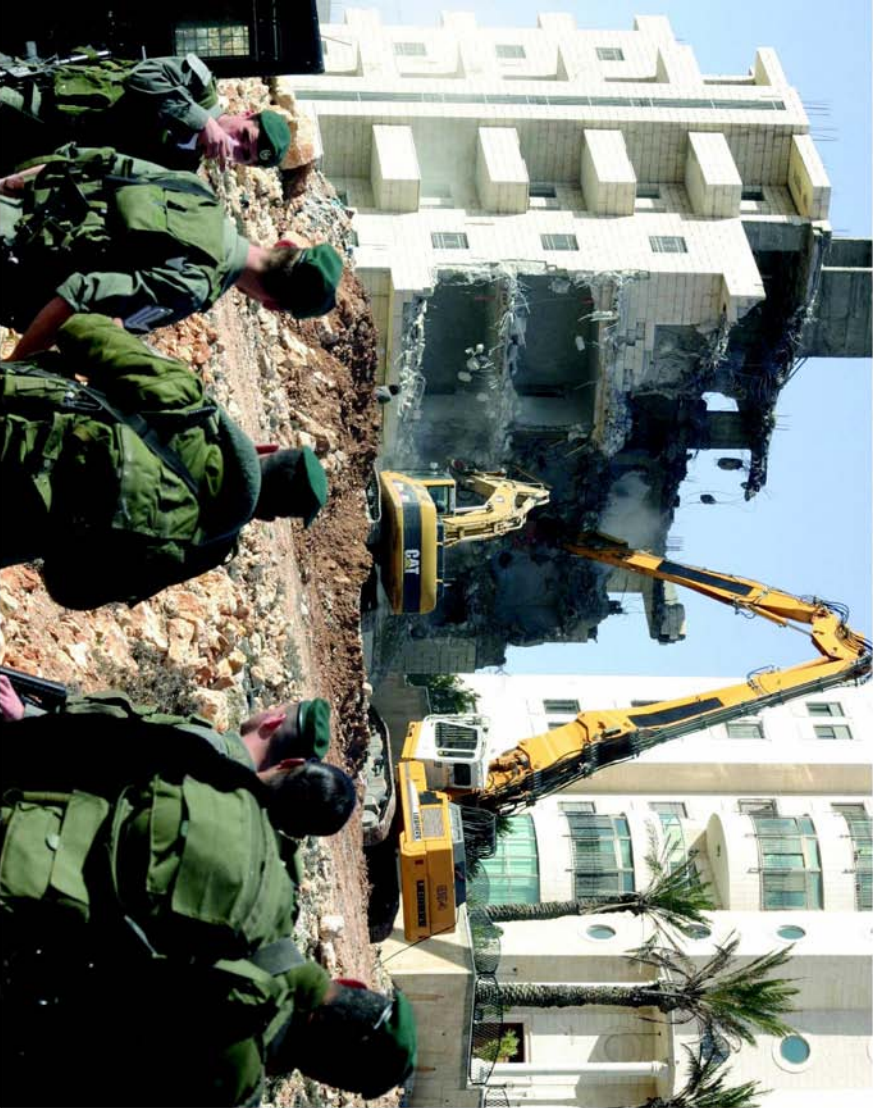
Beit Hanina home, in April 2006. At this point, the building received a stop demolition order, and half the building remained standing but uninhabitable. © Mahfouz Abu-Turk
