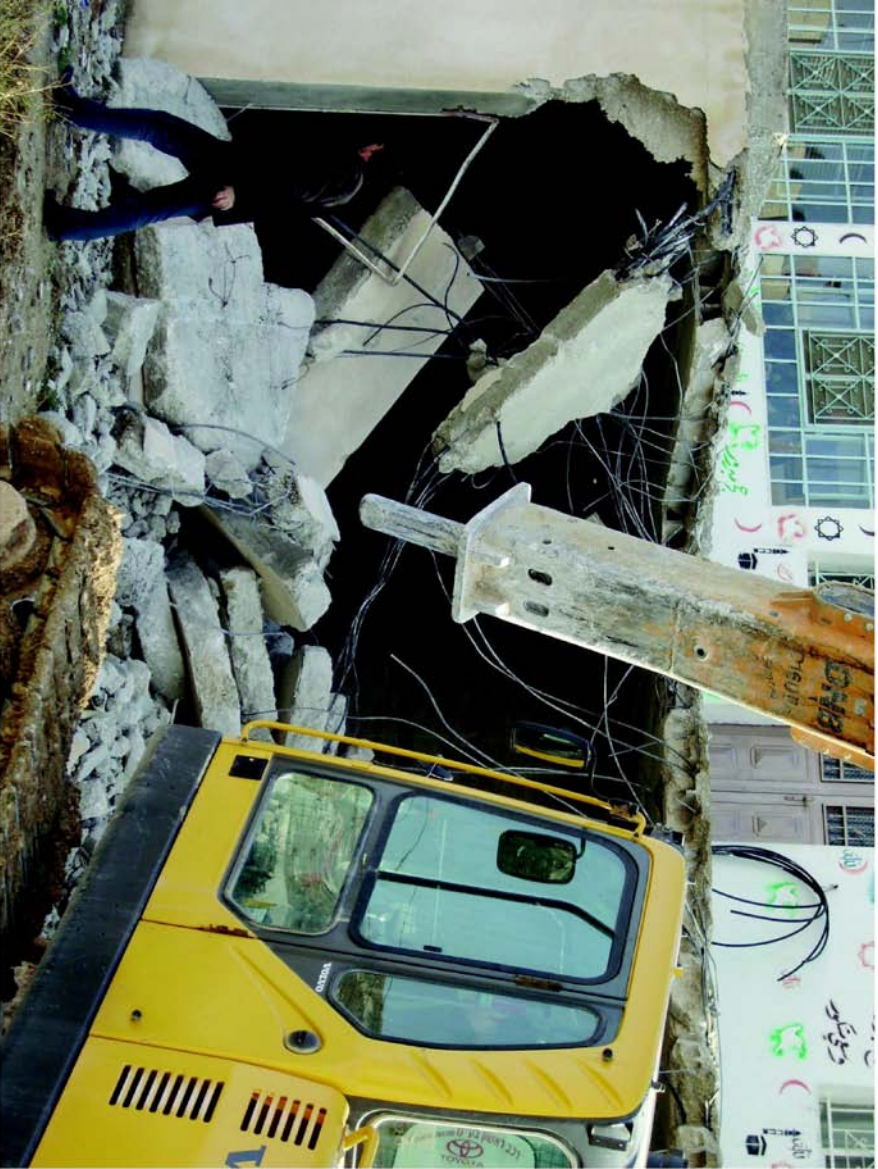
Silvan demolition in 2006 of terminal cancer patient who has since died. It also damaged the building behind. © Godfrey
